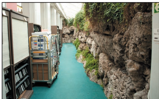
Figure 1. Tufa wall in the Winter Gardens, at County Hall, Matlock (photo: University of Derby).
