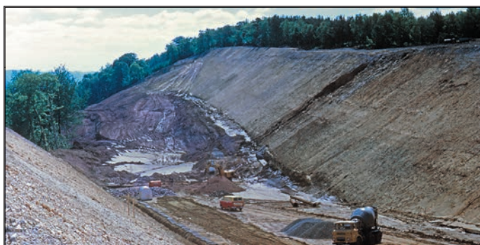
Figure 9. Excavation for a cutting along the re-aligned A38 (Exeter-Plymouth) road, after torrential rain created the gully in the cut slope to expose a complete section through the local sequence of the Upper Greensand.
